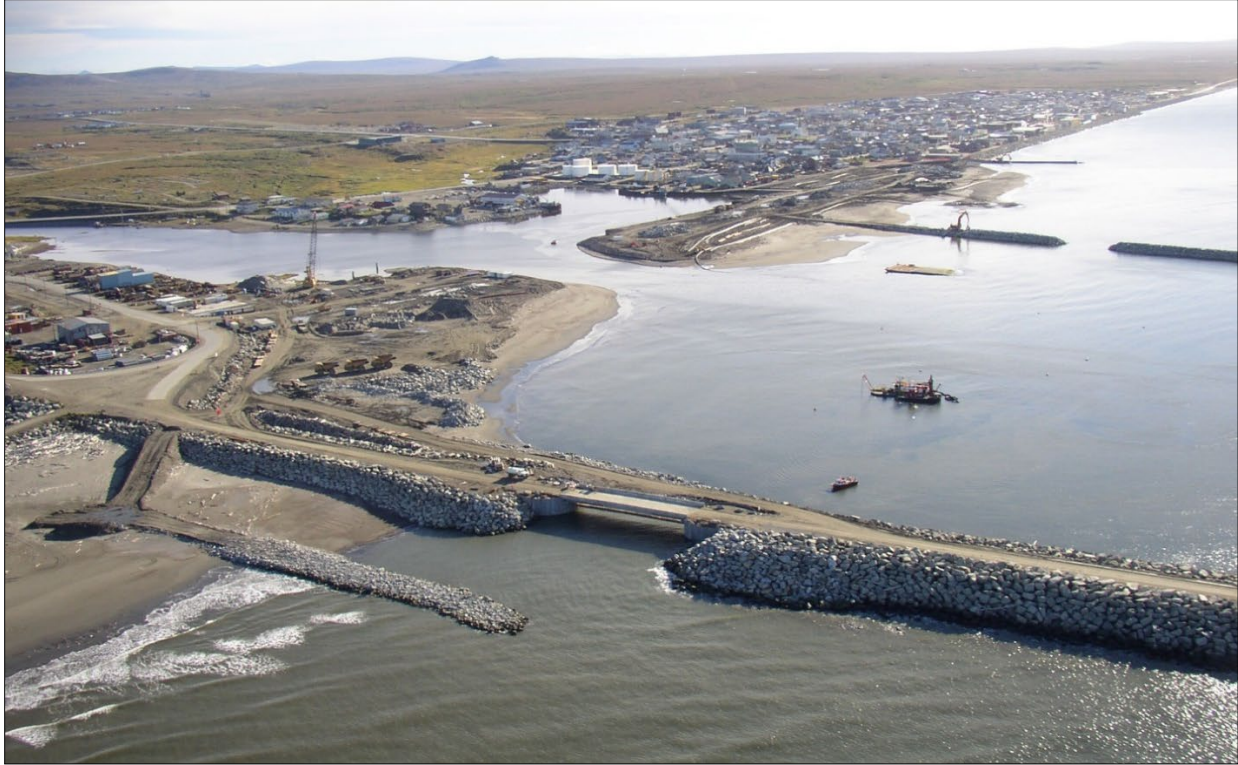
Figure 4. Oblique view of temporary groin and road during bridge reconstruction in 2005 (Photo courtesy of City of Nome).
