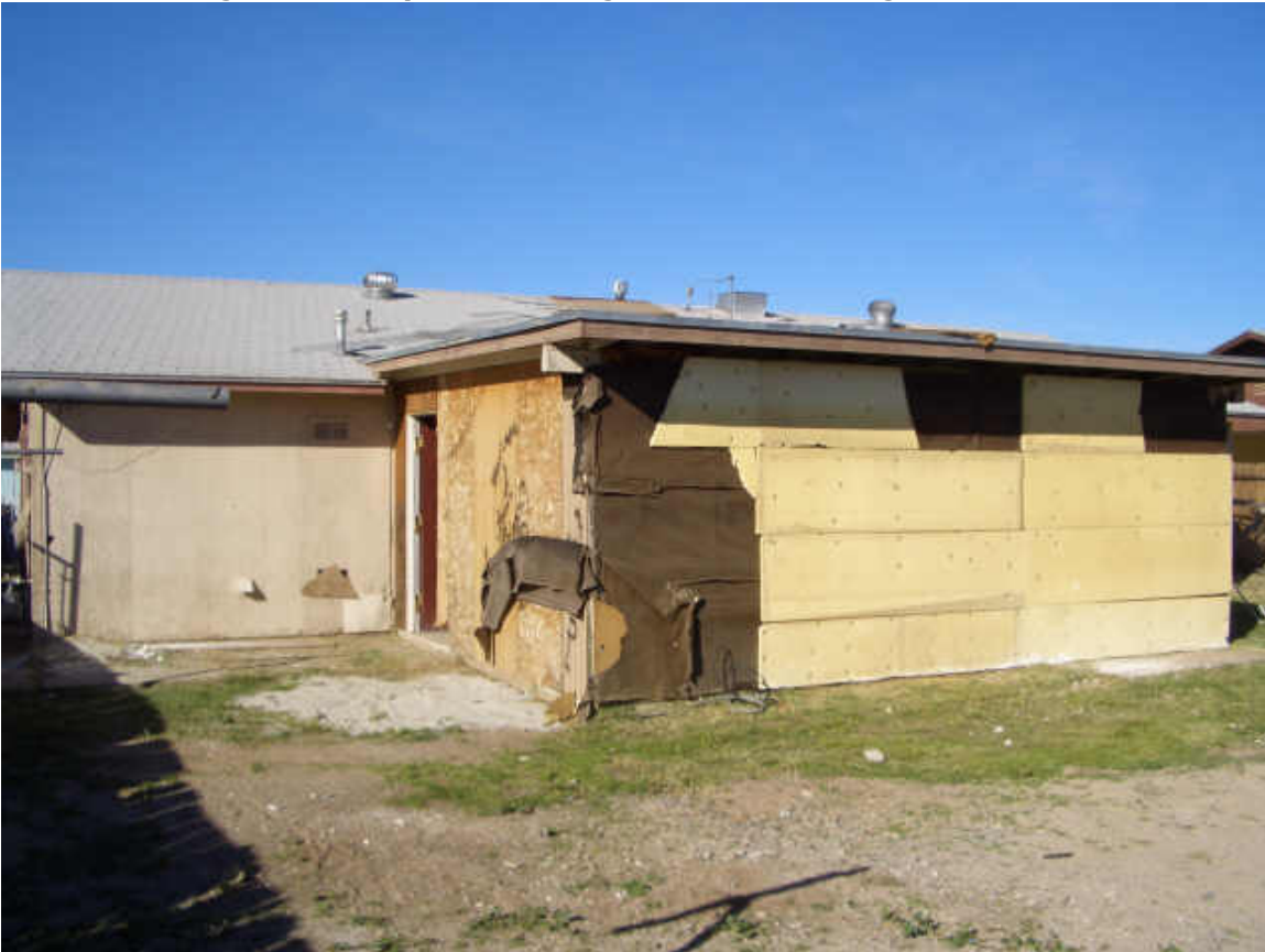
Figure 1 Example of a zoning violation involving a structure.
